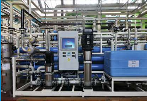
MEMSEP engineers innovative solutions for water treatment plants, tailored to its clients' requirements
